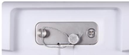
Locked with Wire Seal
